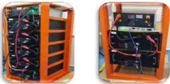
Energy Storage System (ESS)
